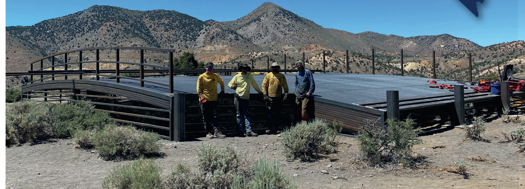
Environmental Protection Services' owner and work crew standing next to a large wildlife-compatible structure constructed, under contract with the Division, over the historic Forman Shaft in Virginia City, Storey County.
